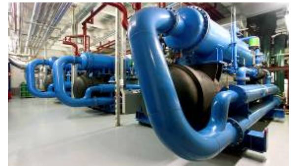
30 MW cooling capacity
