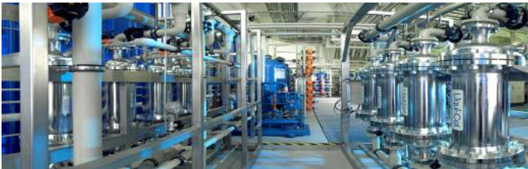
80 m 3 /h Ultra Pure Water Plant
